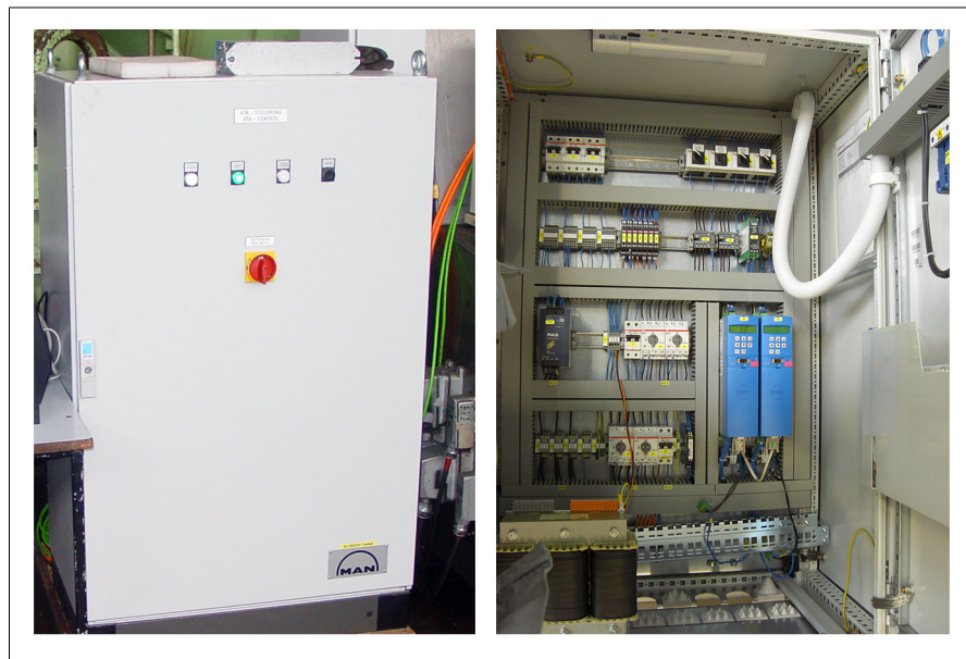
Figure 1: Control Cabinet – VTA control system (VCS)
