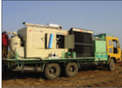
High Pressure water well package powered by Cummins KTA-1150-C
