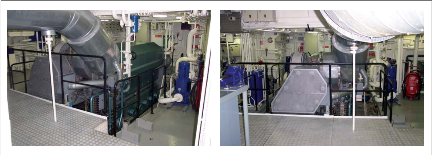
Figs. 6 and 7 M/V MARK AMAY engine room – very clean and well maintained
