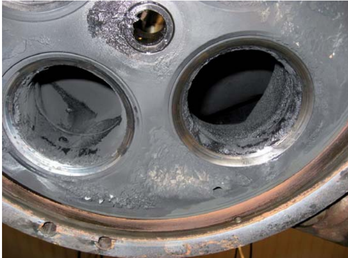
Fig. 11: Cylinder head inlet – and exhaust ring. Coke deposit limited after 26,300 hrs of operation
