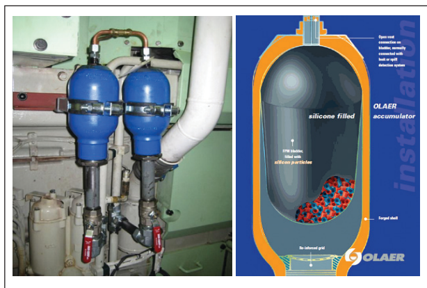
Fig. 7: Gas dampers being tested in service (L21/31 and L27/38)
