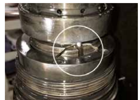
Fig. 71: Wrong assembly of fuel valve part and pump barrel
