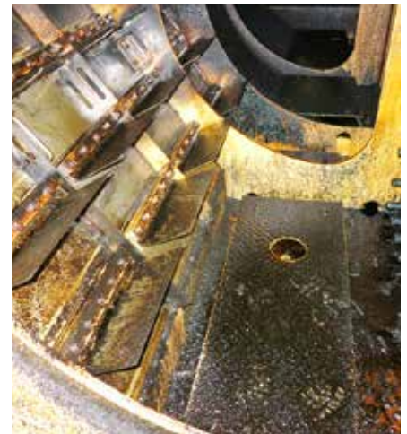
Fig. 84: Sludge and dirt accumulation in the scavenging receiver when operating with EGR
