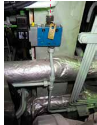
Pneumatic 3/2-way solenoid valve controlled by the ECS
