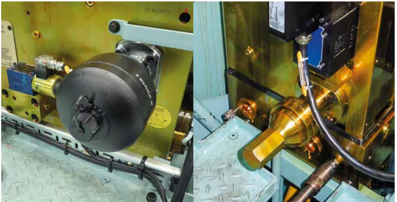
Fig. 3: Left: New 0.7 L accumulator, right: Old 0.2 L accumulator
