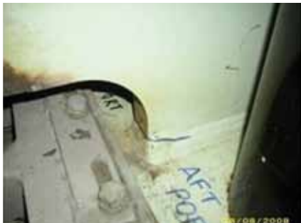
Fig. 35: Lifting bracket cracks
