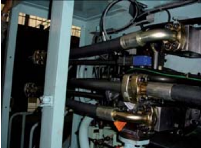
Fig. 28: Flexible hoses on K98
