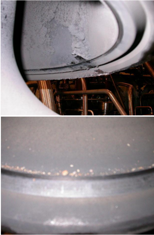
Figure 10: Photographs of the valve spindle and seat ring surfaces after 1,000 hours [6].
