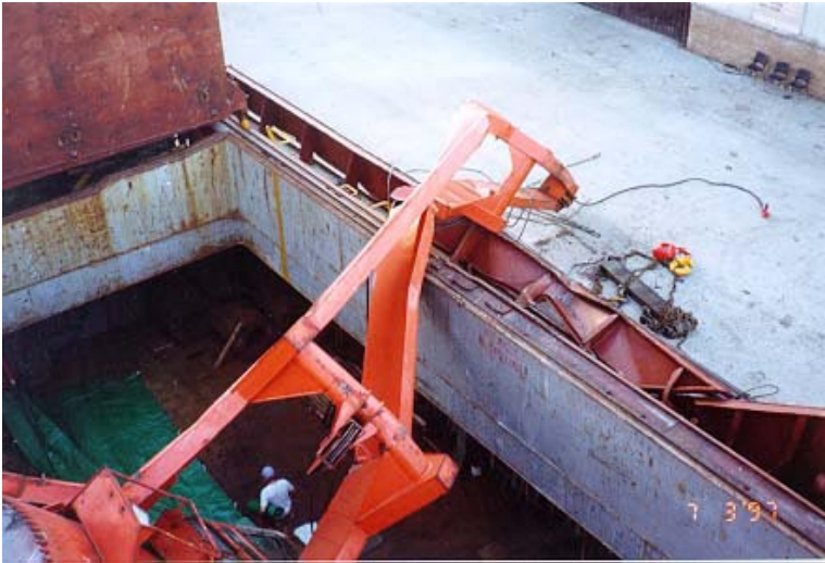
Jib of no. 1 crane lying over the port side of the vessel
