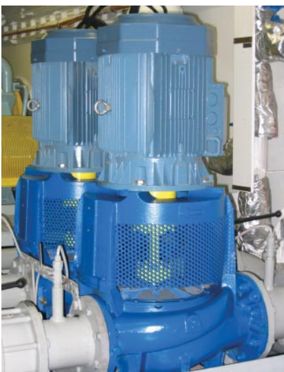
C2G cooling pumps installed onboard, Color Line's 'Color Fantasy'
